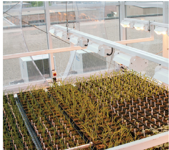
Lighting Control in the Greenhouse
